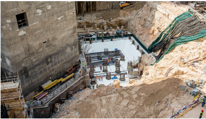
■ The site undergoes a rigid protocol of method statements and risk assessments.
