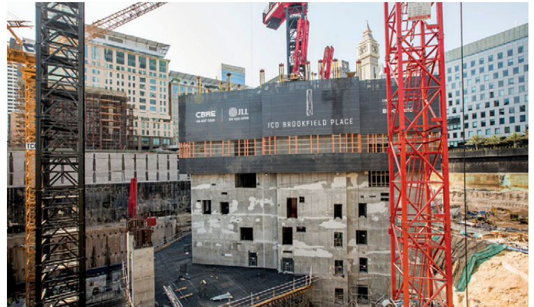
The Favco M2480D crane was shipped in from Australia for the project.
